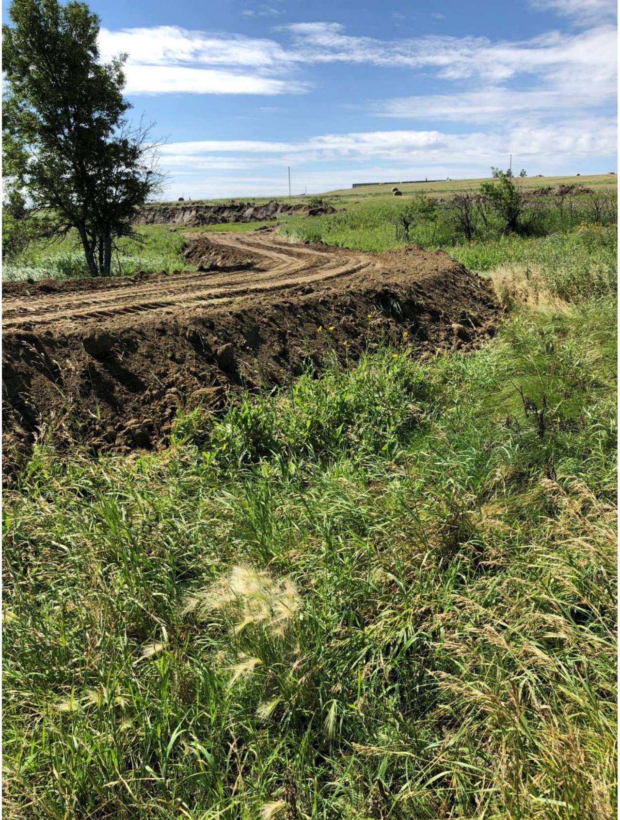
Figure 8: A temporary topsoil bridge was constructed in a saturated portion of the mine.
