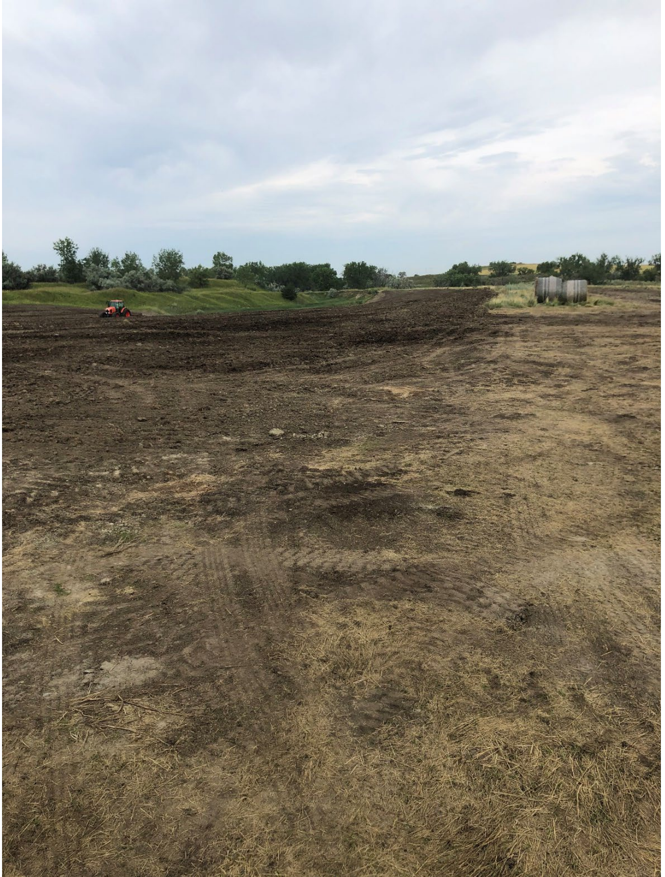
Figure 17: Seeding the reclaimed highwall with a native grass mix in the East Youngtown Tract.
