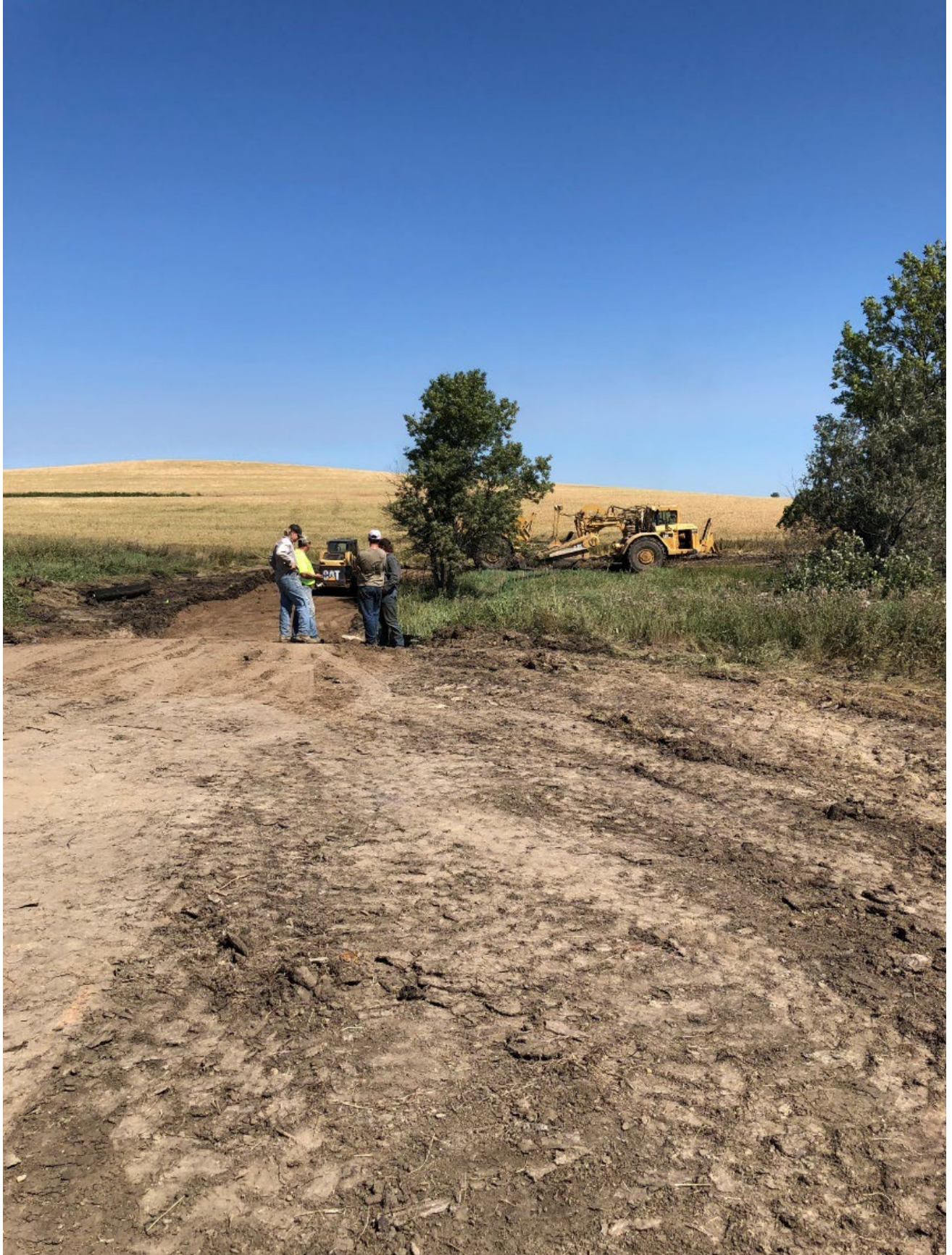
Figure 12: The contractor is using a scraper to haul topsoil in the West Youngtown Tract.
